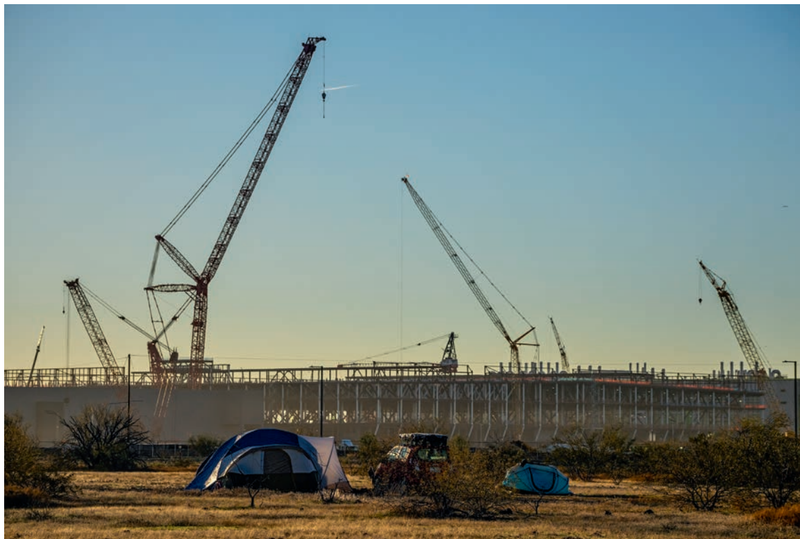
The Taiwan Semiconductor construction site in northern Phoenix. Its three plants will employ 6,000 people—and consume billions of gallons of the city's water every year.
